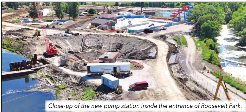
New pump station facing south.
